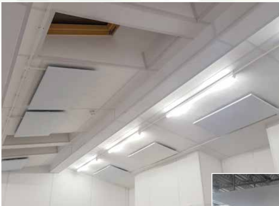
RP radiant panels ceiling mounted in a cricket pavilion in Essex
