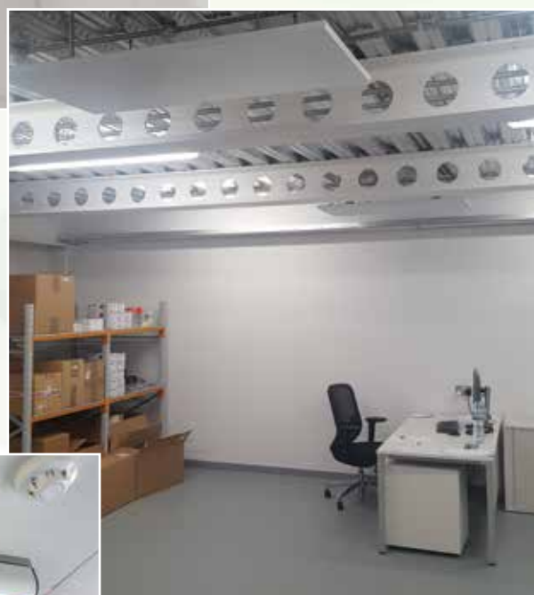
RPs providing unobtrusive heating in a prestige British sportscar facility
